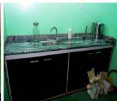
Sluce room with wash hand basin
